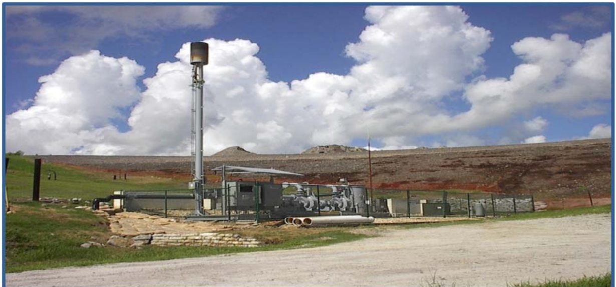
Closed Landfill Gas Flare
